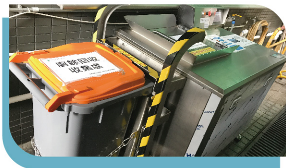
▲ 裝設廚餘機以收集單位的廚餘。 Installation of a food decomposer to collect kitchen waste from different units.
